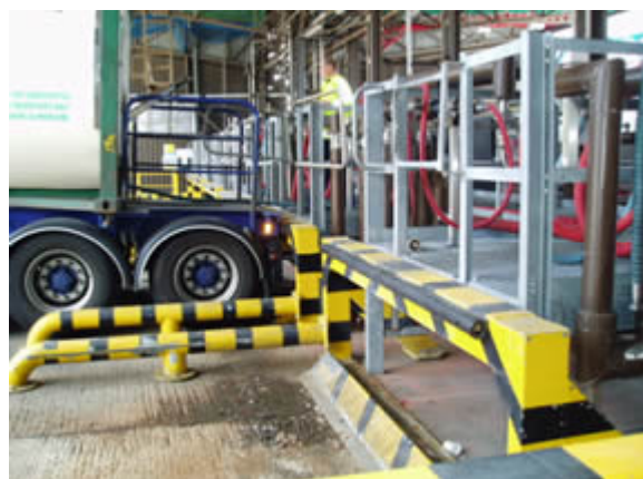
Figure 2 – tanker in the loading bay
